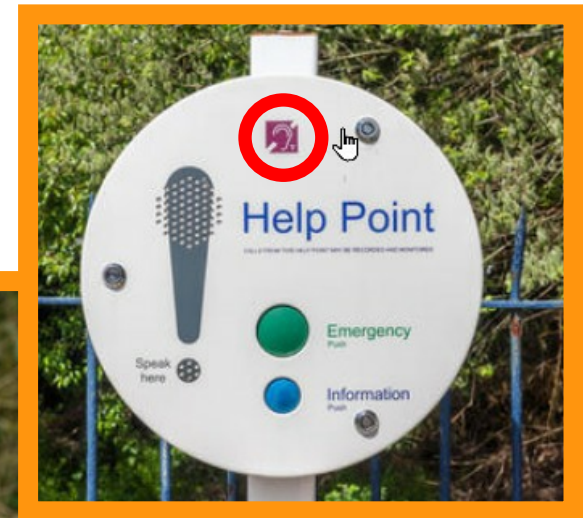
Looped emergency help point in parking
